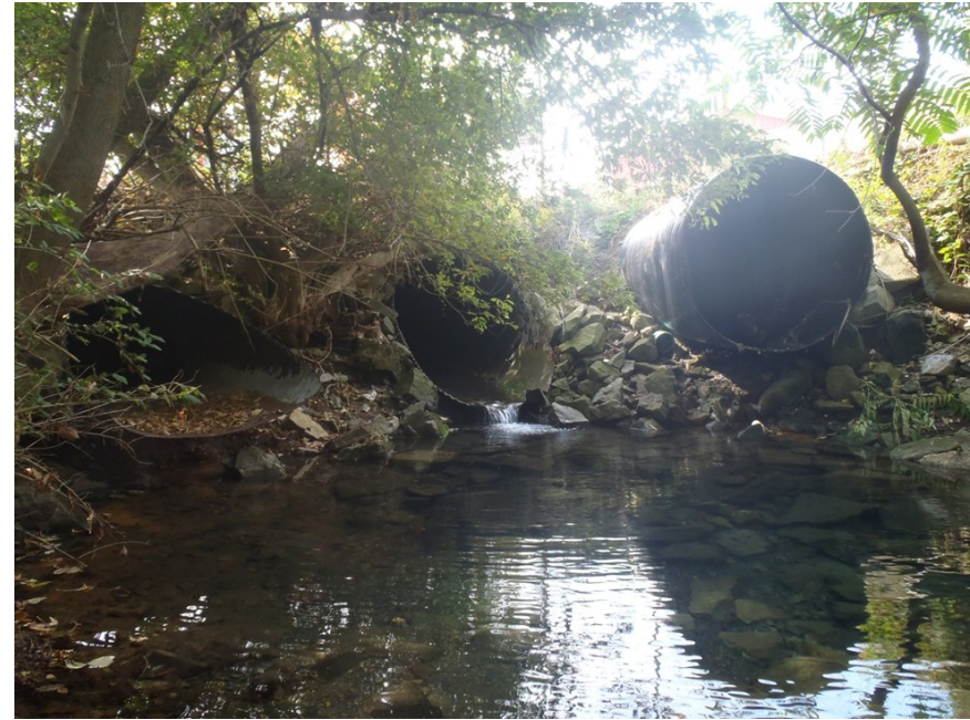
Three storm drains located above the Duck Pond. The two furthest right pipes drain the Downtown and Main Campus area, respectively.
