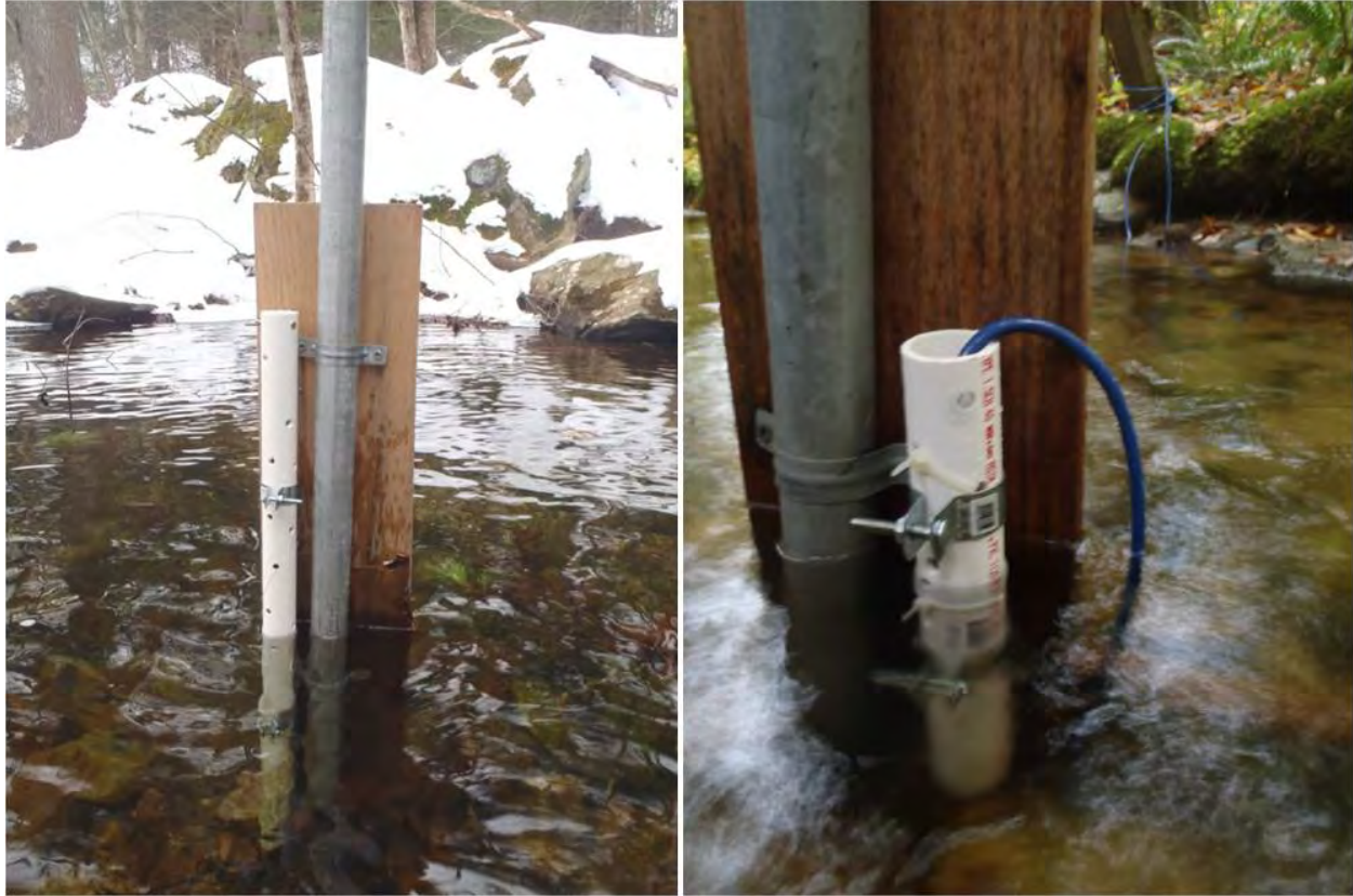
Figure 25. Non-vented (left) and vented (right) pressure transducers attached to staff gage board using conduit hangars.
