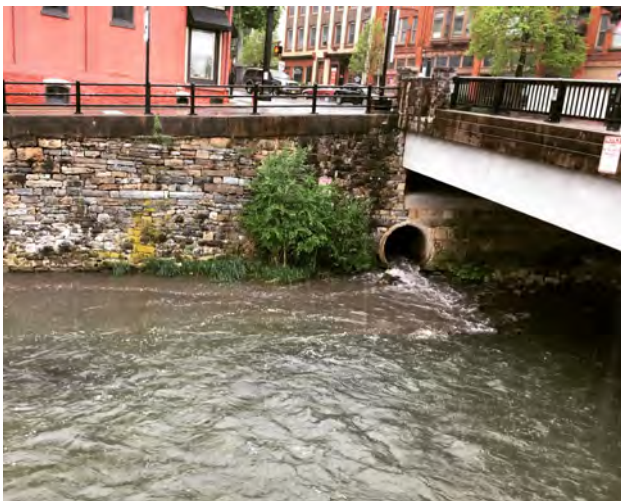
Fig. 4 A storm drain releasing surface runoff directly into Spring Creek
