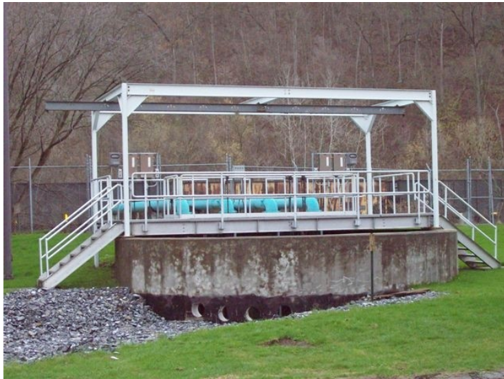
Dewatering tank at Bellefonte Wastewater Treatment Plant (credit: T. Smith)
