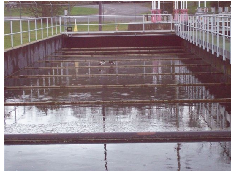
Bellefonte Wastewater Treatment Plant's final clarifier system (credit: T. Smith)
