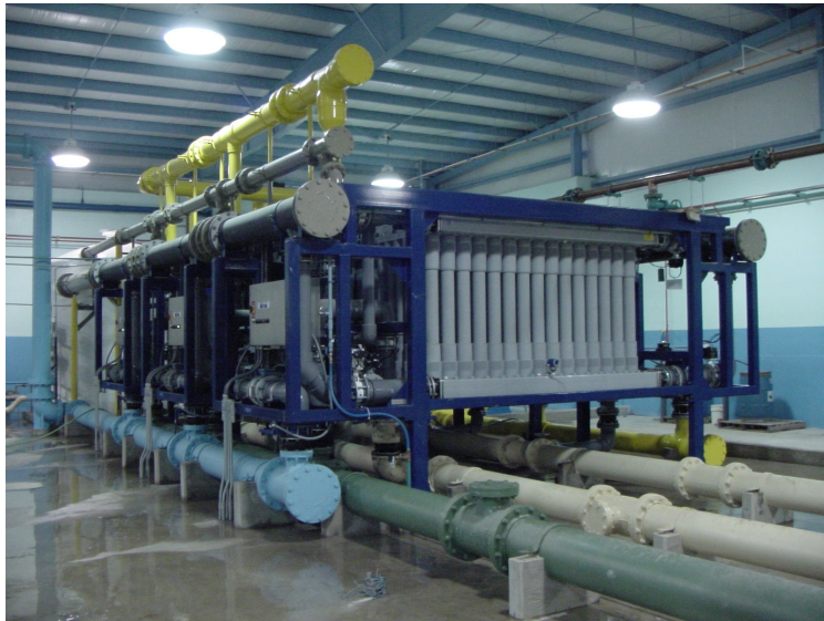
University Area Joint Authority's Advanced Water Treatment (AWT) facility (credit: J. Brown)
