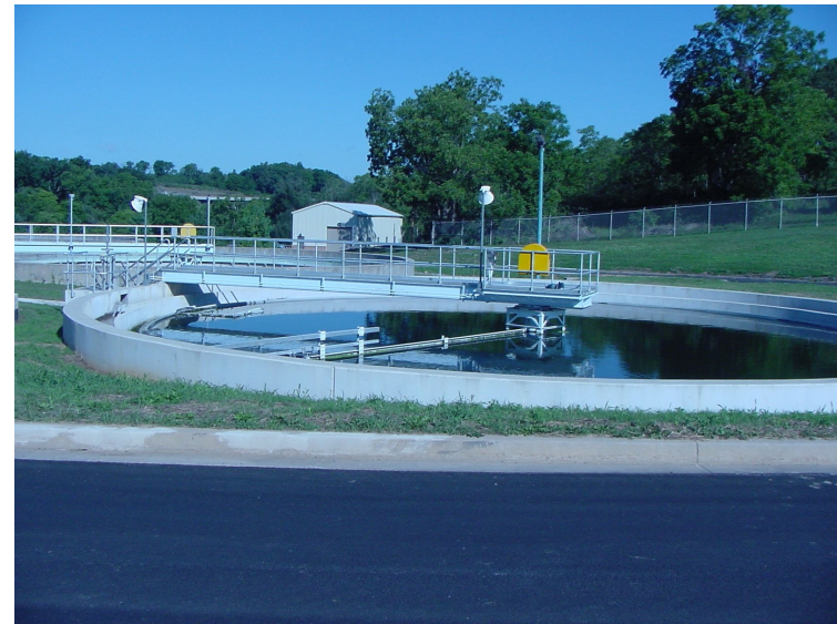
UAJA's secondary clarifiers (credit: J. Brown)
