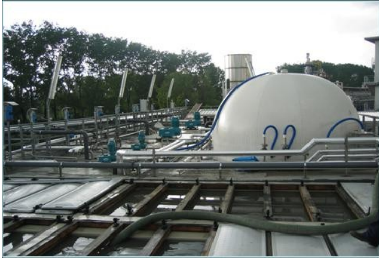
Anaerobic biological treatment tank (credit: Austep SRL)
