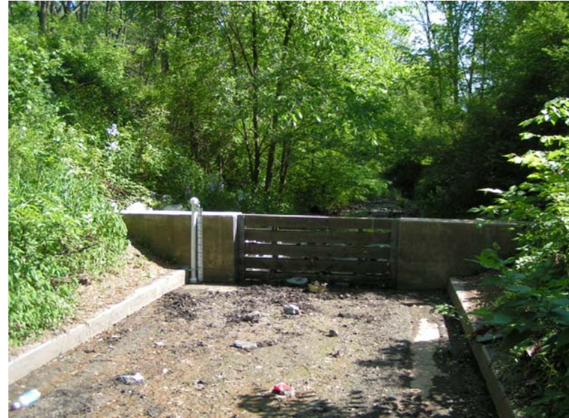
Debris collector constructed downstream of a storm water conveyance in State College Borough (credit: G. Smith)
