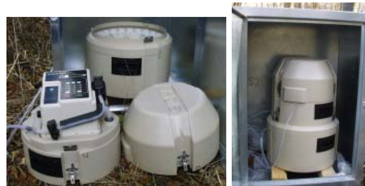
Figure 17 & 18. Storm-water equipment located at each site. Photos: R. Dunlap
