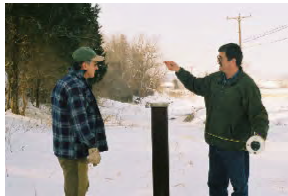
Figure 16. Bryce Boyer, WRMP volunteer, and Mark Ralston, WRMP committee member, install ground-water monitoring equipment at Fillmore.
